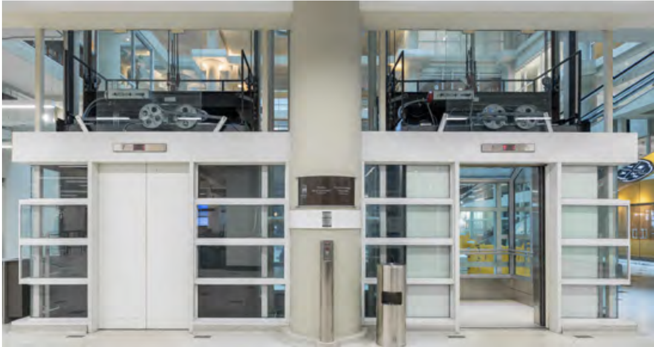
Image Description: The elevators inside Queen's Quay Terminal
